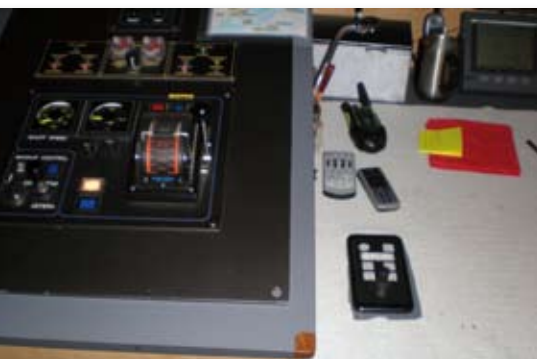
The Joystick Control Unit for the Navigator Pan / Tilt is integrated in the bridge.
