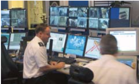
A part of the control room of the Security Operations Center at Copenhagen Airport.
