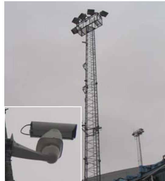
One of the FLIR Systems SR-100 thermal imaging cameras installed on a Pan/Tilt.
