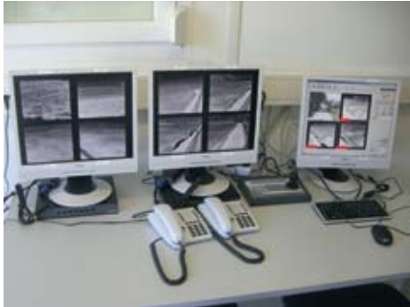
Part of the control room
