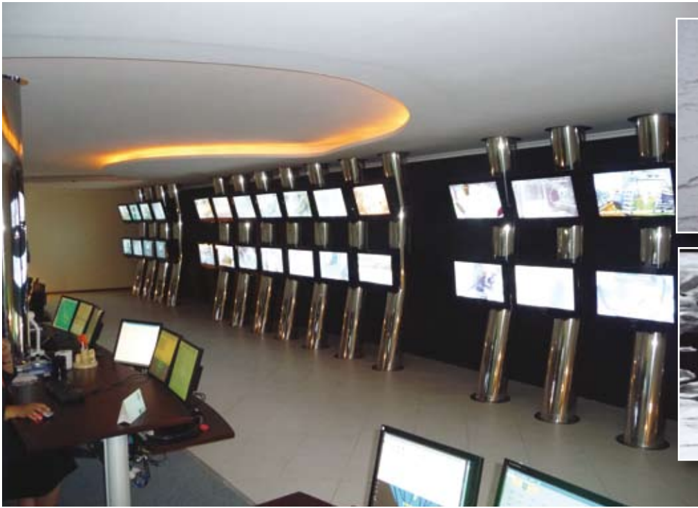
The main control room at Oranjemund.
