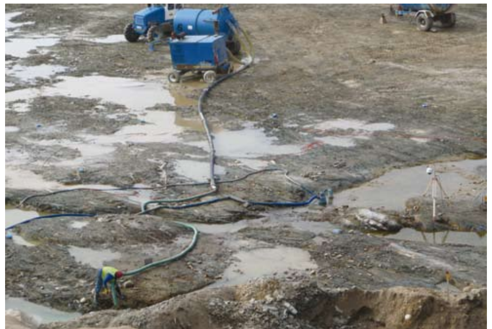
The bedrock is cleaned by workers using a containerized vacuum cleaning system. Note the "Spider camera" standing on the right which is monitoring the worker's activities closely.
