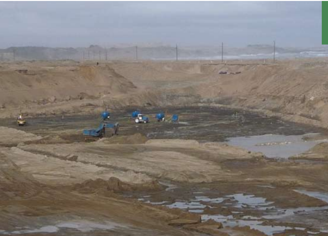
One of the bedrock areas with thermal imaging cameras installed around it.
